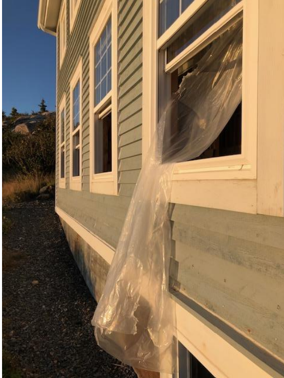
Still photo made from the video taken months earlier. Wind lifting the plastic through open window.
